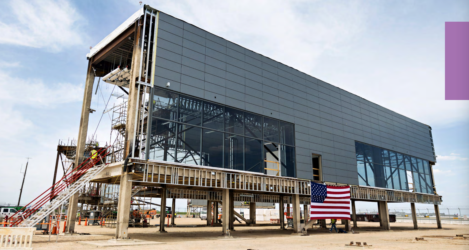
ATLNext projects like the Concourse D Widening project follow a thorough risk management process
